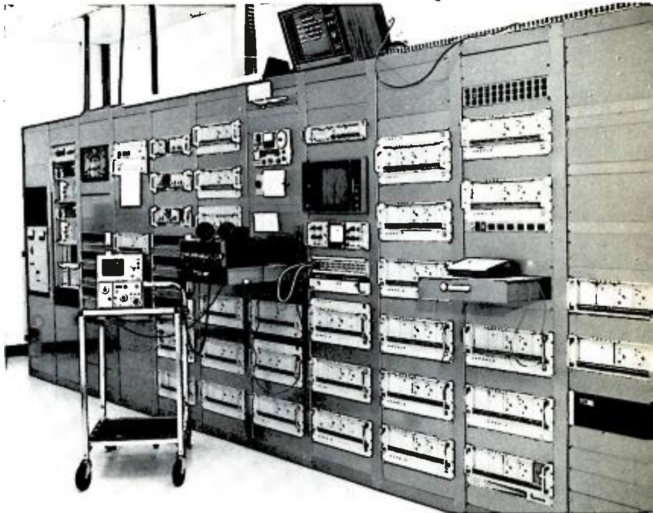
Tulsa Cable's all-Jerrold headend distributes the system's 24 channels to over 21,000 cable subscribers.
